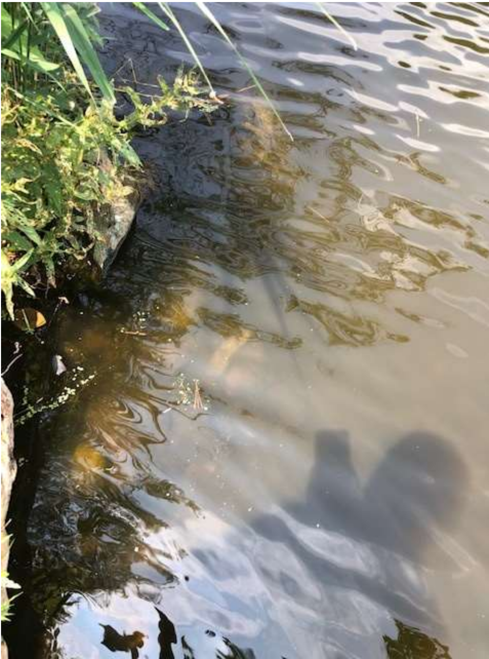
View of stones, concrete and brick fragments immediately adjacent to historic fill pond edge.
