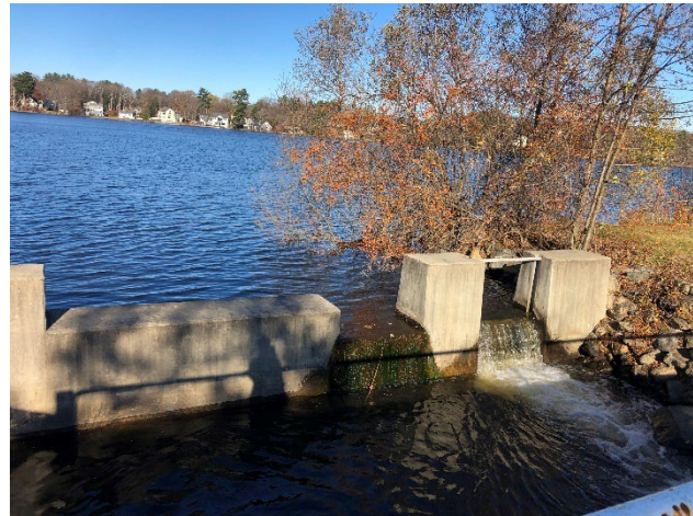
The spillway at Pillings Pond. A stoplog system appears to allow for some level of drawdown. However, deeper drawdown may require coordinated dewatering of the basin just downstream. This would need to be evaluated further to pursue a conventional “dry” dredging project.
