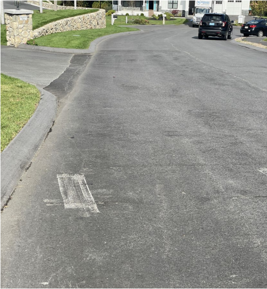
Photo 1. Minor scuffing along roadway
