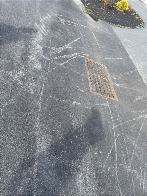
Photo 5. Scuffing along roadway near double catch basin
