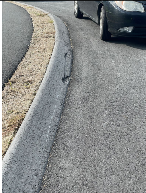
Photo 4. Wear and tear along curb
