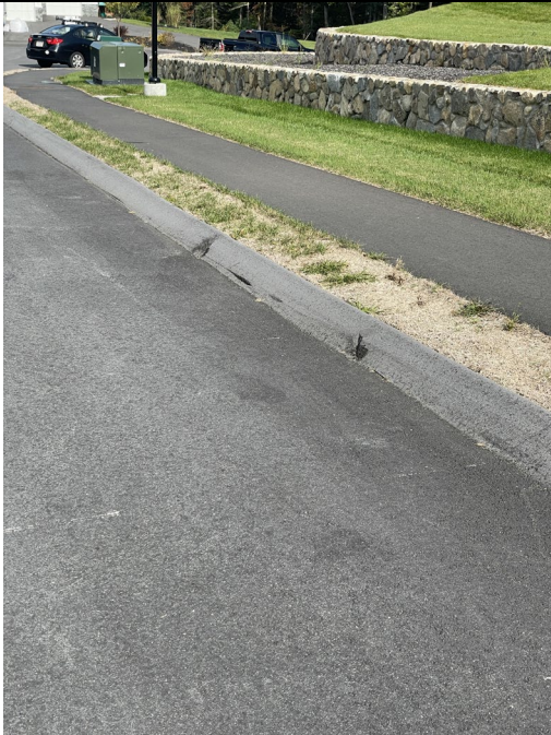
Photo 3. Wear and tear along curb
