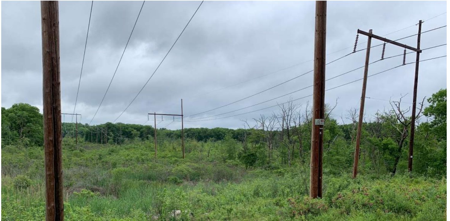
Photo #3: View of the wetland near Structure 82 on both Lines, where the proposed soil boring and work pad are within the 100-foot Buffer Zone to BVW and 200-ft Riverfront Area looking northwest.
