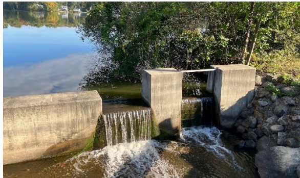
Outlet system at Pillings Pond along Summer Street.
