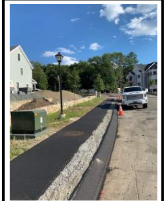
STREET LIGHTS COMPLETE AND OPERATIONAL
