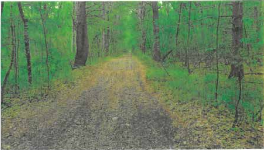
Photo 1. The 1.3-mile abandoned railroad bed in the northern portion of the property makes a good anchor for several of the proposed trail loops. We propose that the surface be re-graded to eliminate the frequent dips and washboard condition. Invasive shrubs and occasional hazard trees should be removed.
