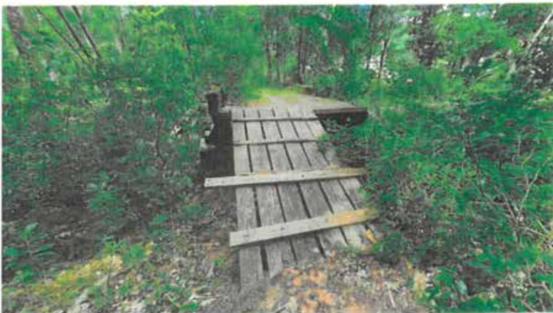
Photo 8. This bridge connects Loop 7 with Elm Street by way of a private property. The bridge itself needs improvements to its abutments.
